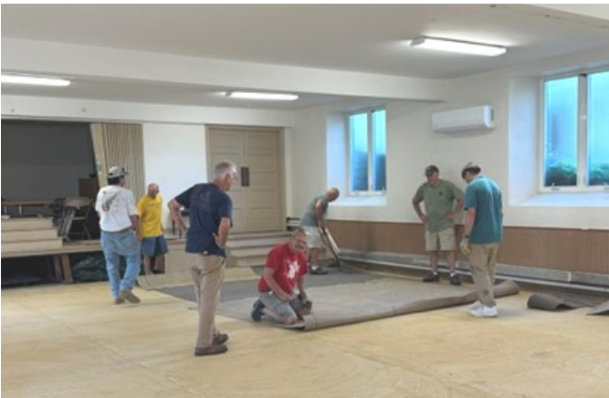
Volunteers remove carpeting. Renovations included new flooring, fresh paint, and other cosmetic upgrades!
